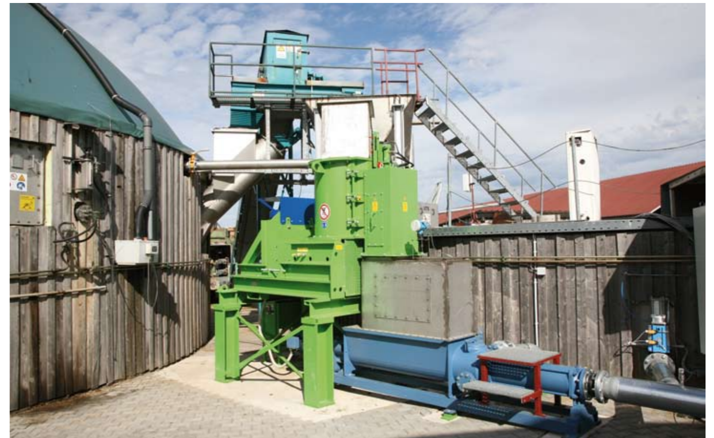
The Bio-QZ along with the Bio-Mix pump has been perfectly integrated into the existing system design.
